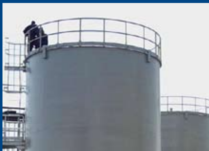
Bio Acid Tanks 5.4m diameter x 7m height Haradh Crude Oil Project - Aramco
